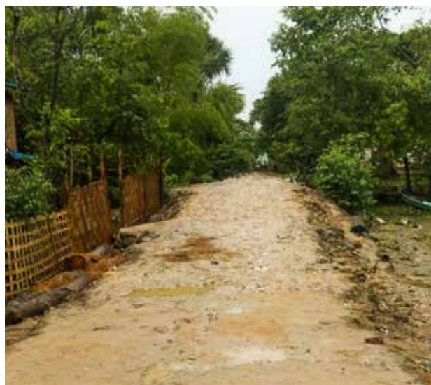
Access roads to schools can be barriers to education for children with disabilities © Myanmar Education Consortium (Myint Maung Maung)
